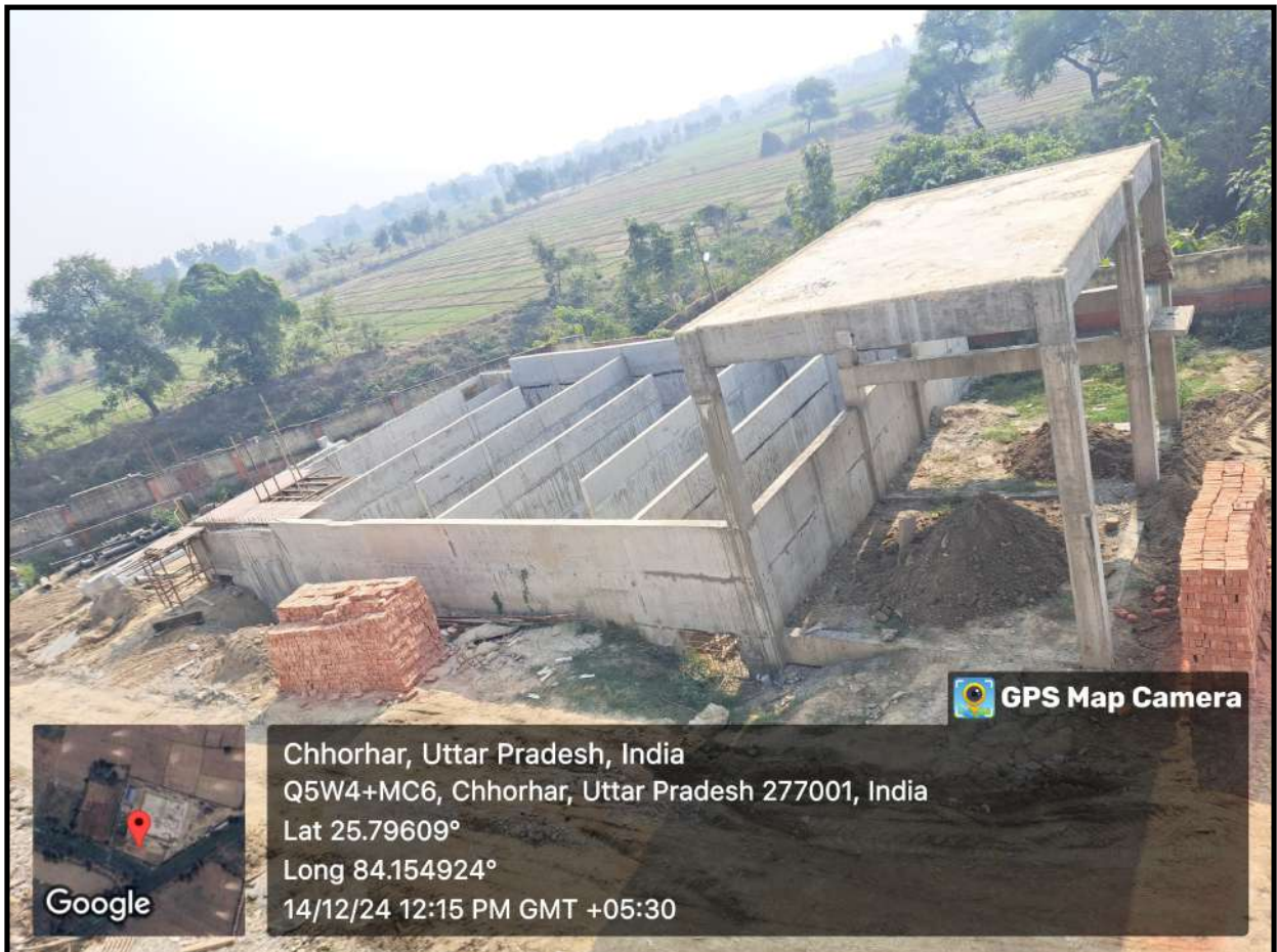
CHLORINE CONTACT UNIT
